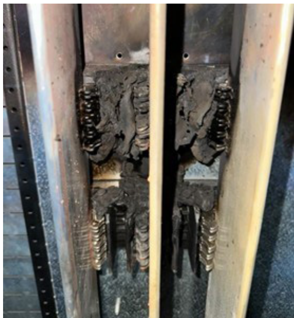
Picture 13. Melted busbar plug.
