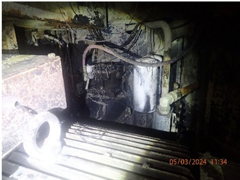
Picture 12. Damaged compressor after fire.
