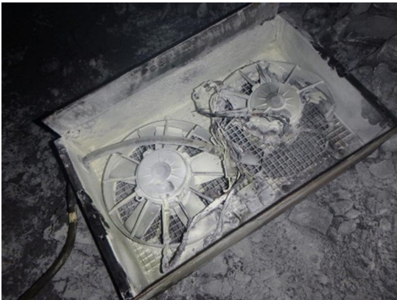
Picture 9. Condenser unit after fire.
