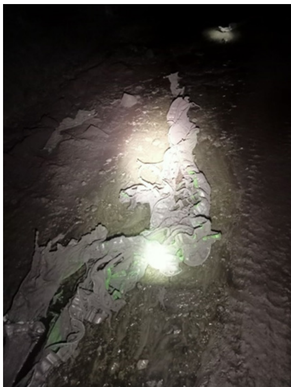
Picture 13. Damaged ventilation bag.
