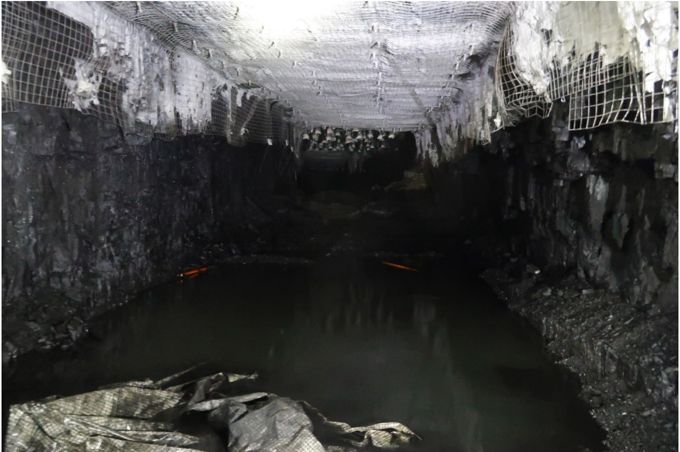
Figure 2: 12 cut-through inbye to intersection at 'Z' heading with floor stripped (for context of final roadway dimensions)
