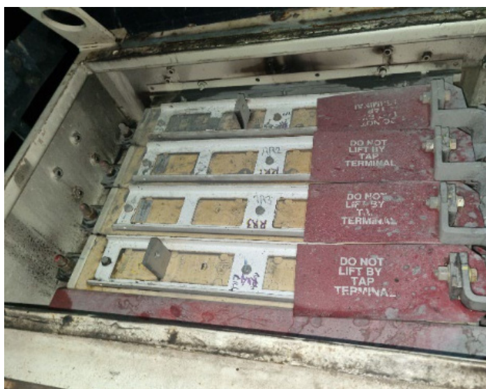
Picture 17: Misaligned grids.
