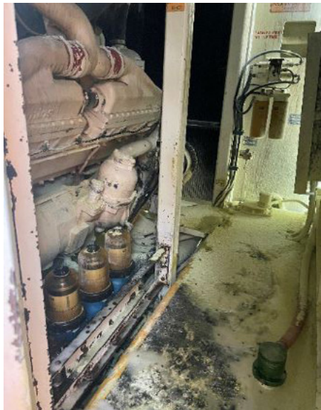
Picture 14. Engine compartment after fire.
