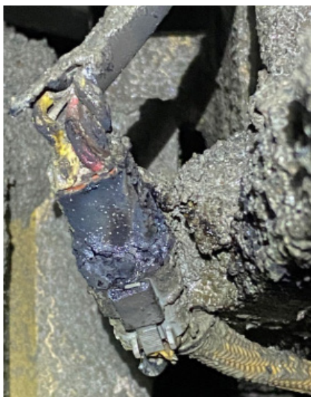
Picture 15. Electrical connector after fire.
