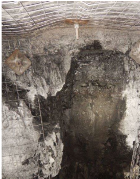
Picture 2. Damaged mesh after rib failure.
