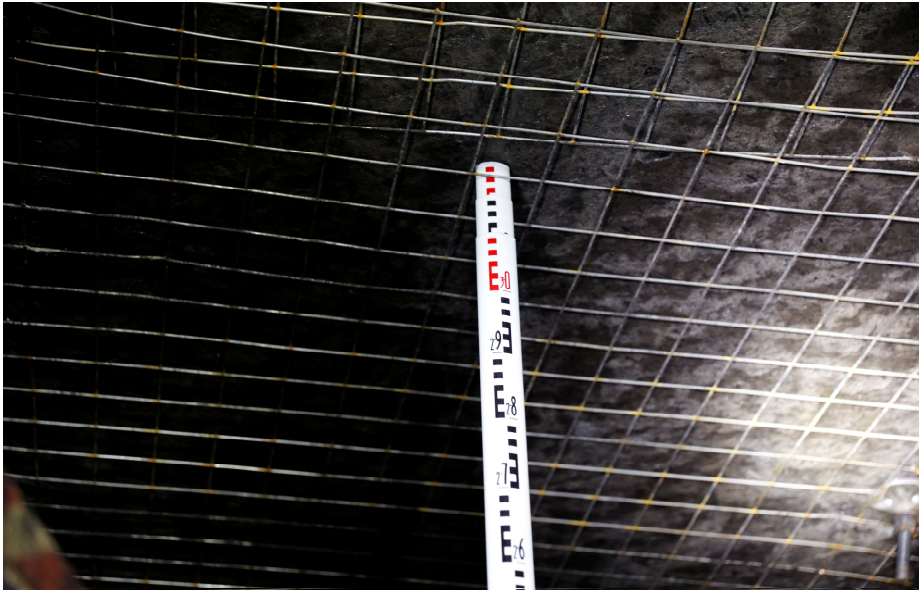
Figure 7 Roof height measured at rear right of the CM boom to be 3.13 metres
