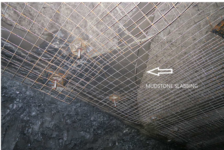
Figure 6 Mudstone roof slabbing supported by mesh and bolts, outbye of incident site
