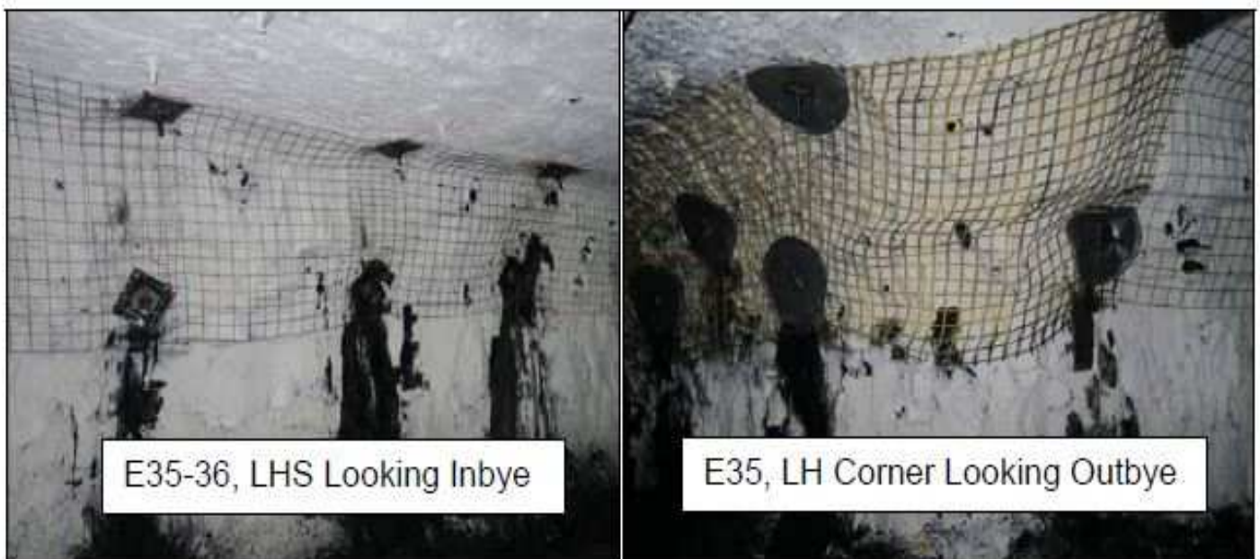
Figure 12 Upper rib support observed by investigators in 821 panel
