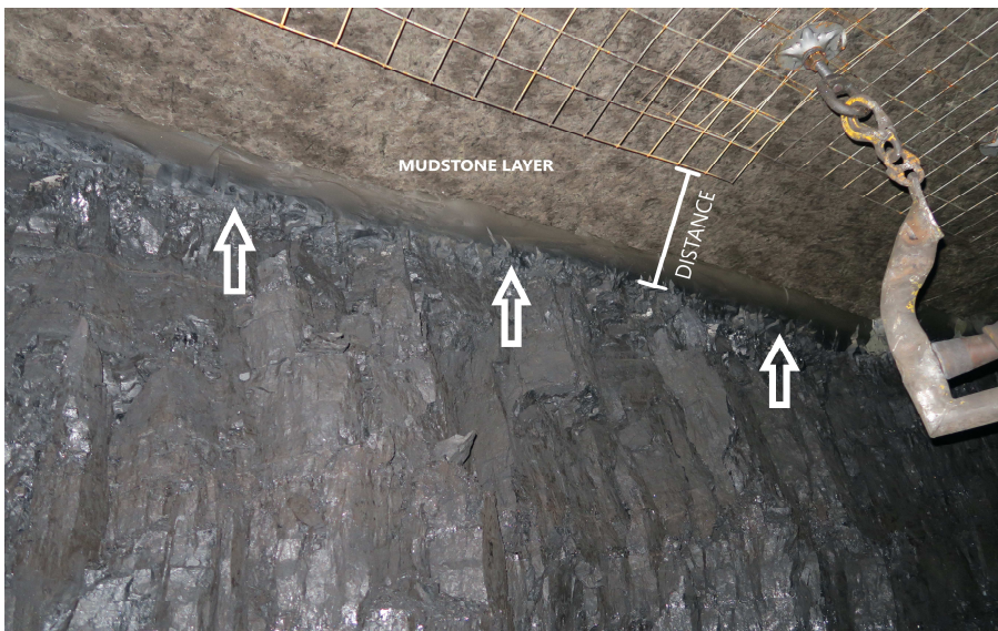
Figure 5 Mudstone layer between coal and sandstone roof at incident site and mesh sheets
