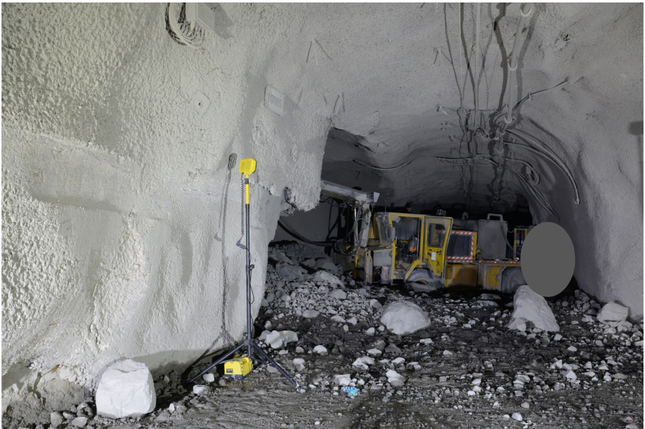
Photograph of the mobile plant and drive taken by an Investigator on 8 September 2015 (after recovery of deceased worker). Photograph taken from north of underground drive looking south.
